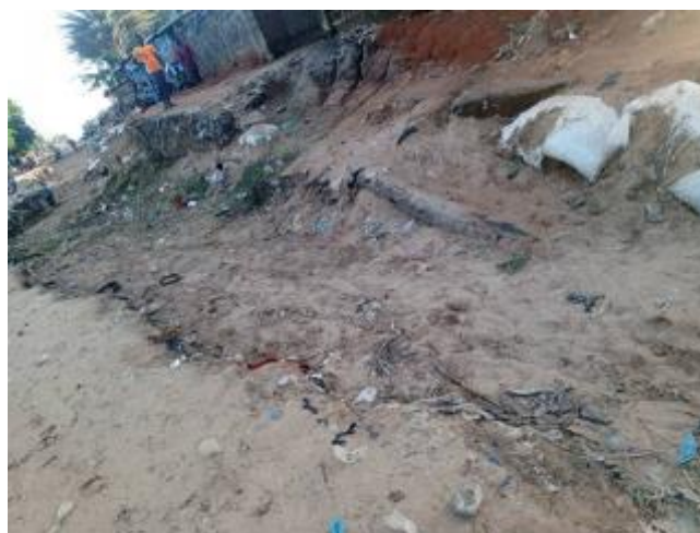
Figure 8: Partial view of a road degraded after the floods in Malanville
