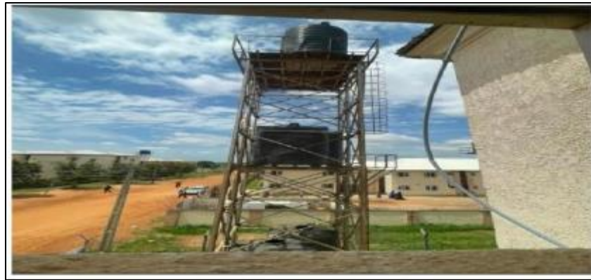
Figure 8: Rain tanks / cisterns as a water harvesting strategy, New Boys Hostel (Chief Set)
