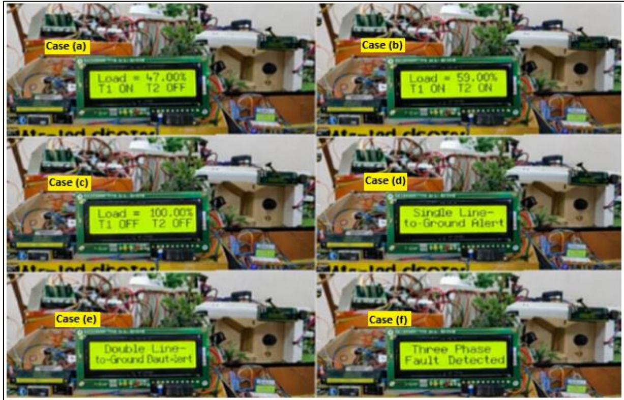
Figure 11 Real-time operational responses of the proposed Arduino-based smart power system under various load and fault conditions:
