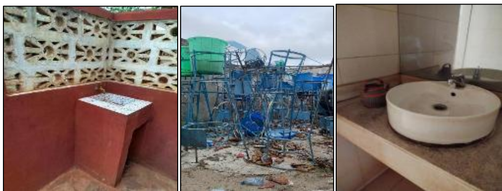
Figure 1 Handwashing facilities in schools of Abomey-Calavi [CEG Le Méridien de Cocotomey (image 1), CEG Allada (image 2), Lycée ASBA/Akassato (image 3)]
