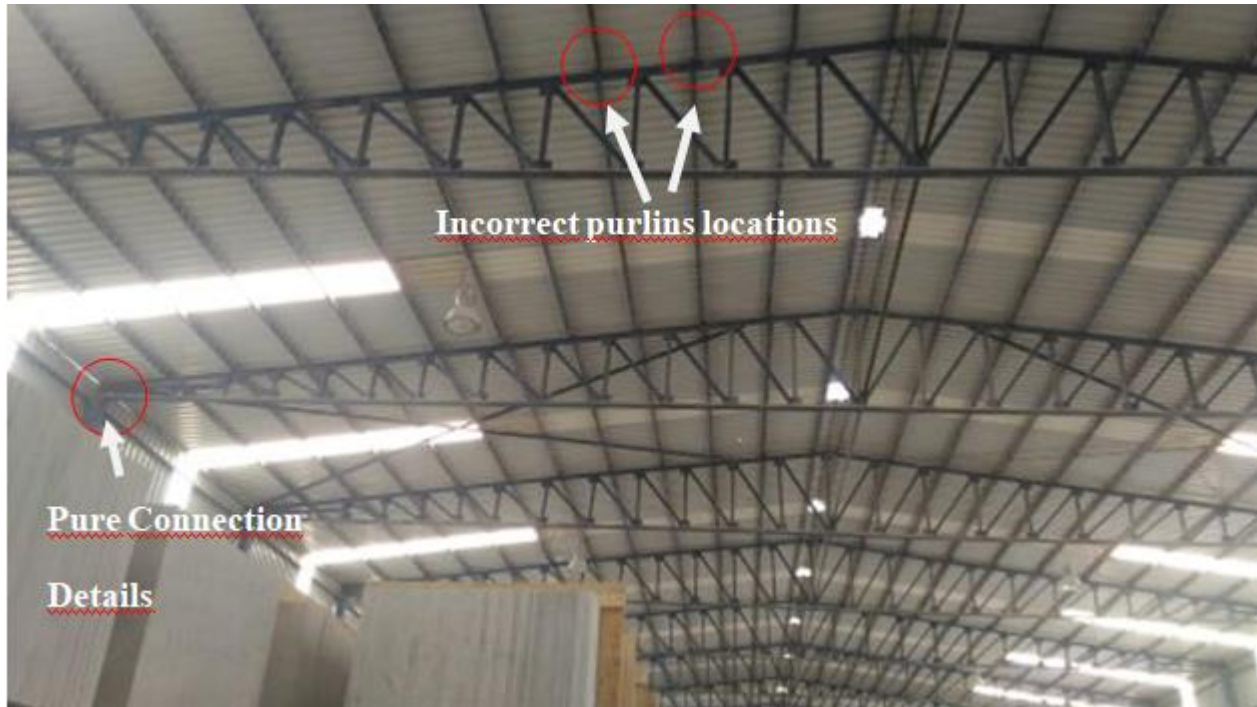
Figure 2 Incorrect supporting of purlins on the steel trusses
