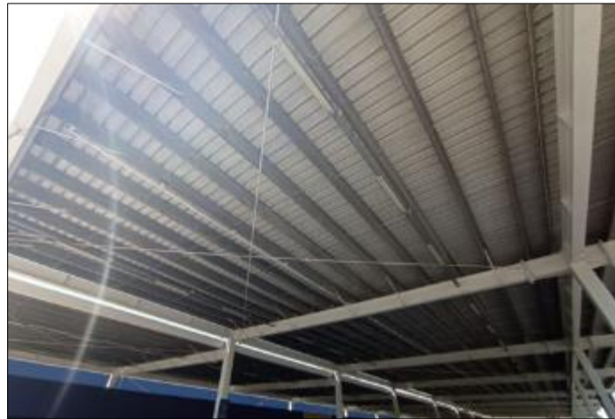
Figure 3 Weak roof bracing
