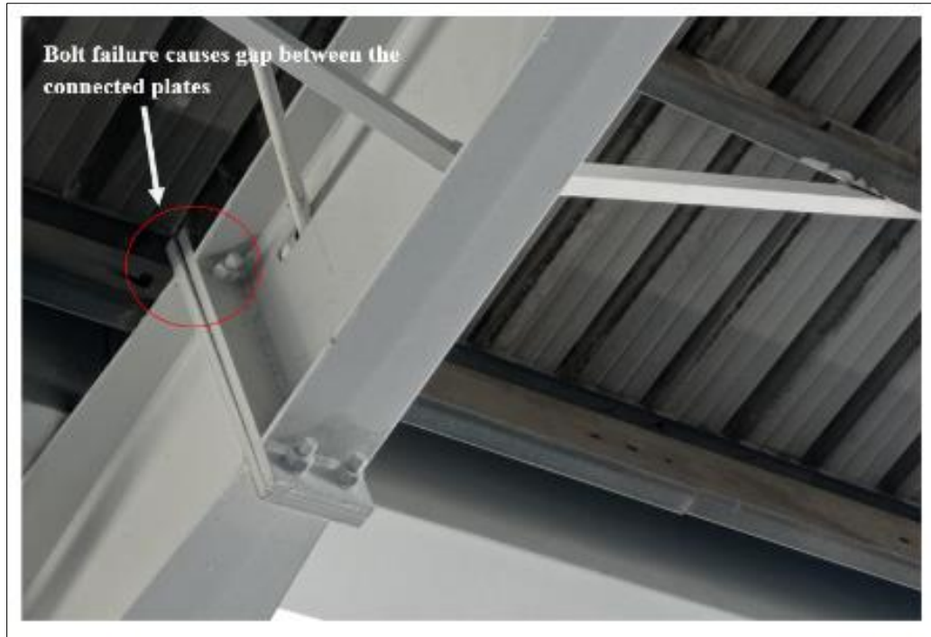
Figure 6 Inadequate number of bolts or incorrect choice of bolt materials
