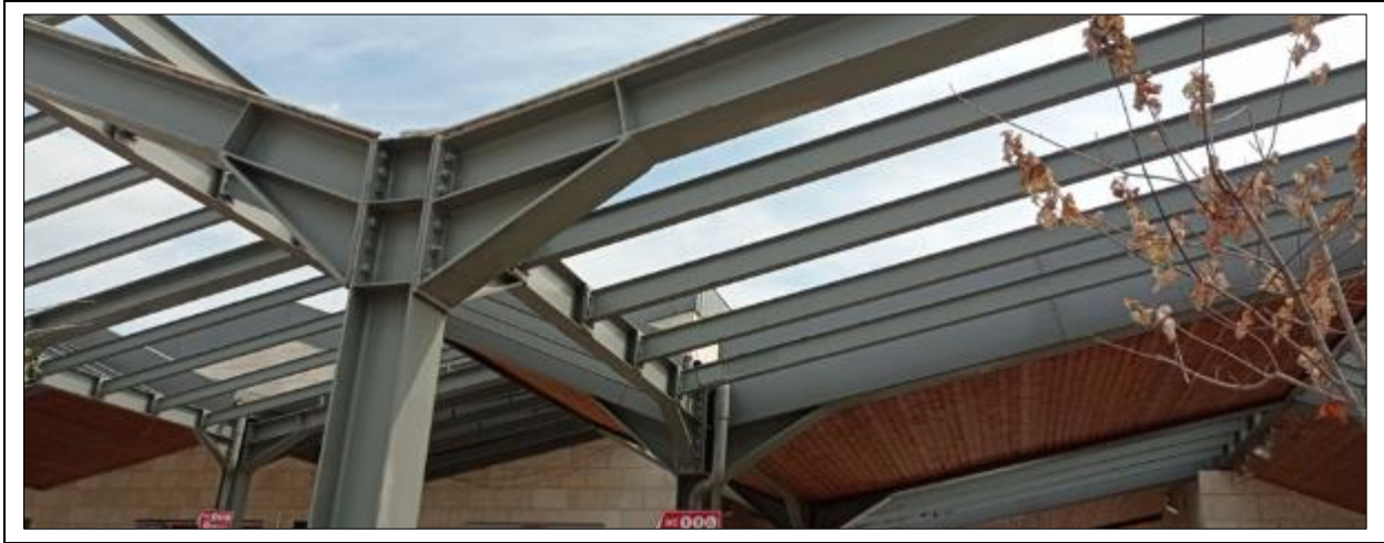
Figure 8 Over-designed structure due to over estimation of loads
