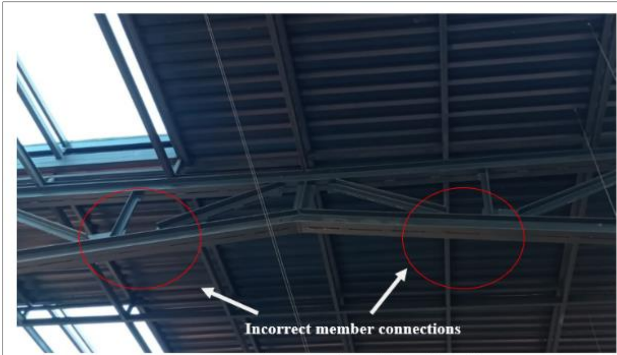
Figure 4 Incorrect connections of roof truss diagonal members
