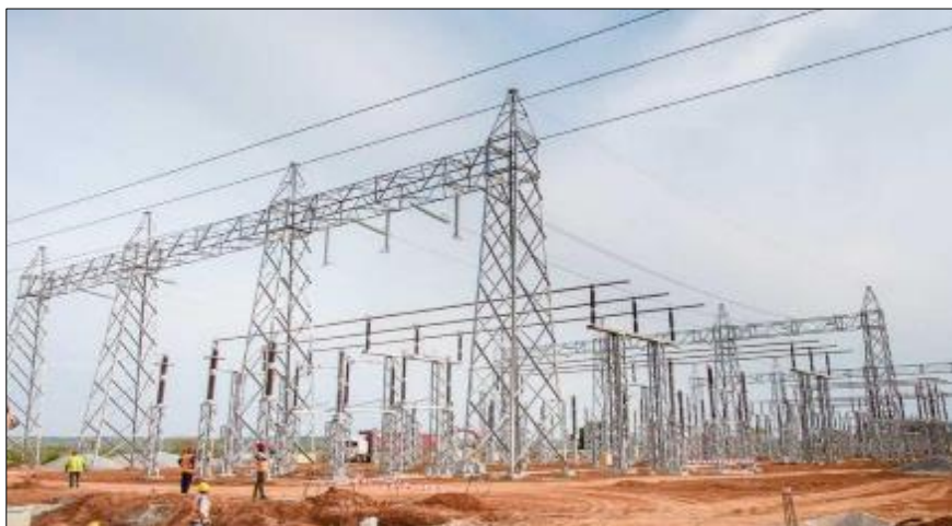
Figure 3 Electrical Grid Infrastructure (Google Photos)
