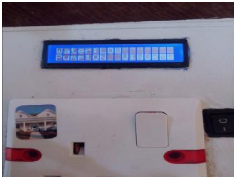
Figure 15 Testing of the Low State of the Water Level Control System
