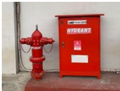
Figure 2 Hidran at PT Wijaya Karya Beton Tbk. Pasuruan
