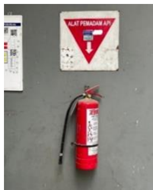
Figure 1 Fire extinguisher at PT Wijaya Karya Beton Tbk. Pasuruan
