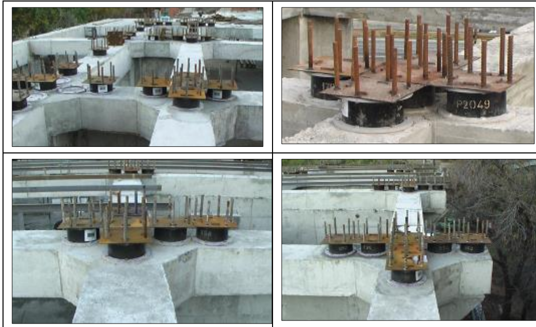
Figure 4 Examples on installation of rubber bearings' clusters in the 16- and 14-story base isolated apartment buildings of multifunctional residential complex "Arami"
