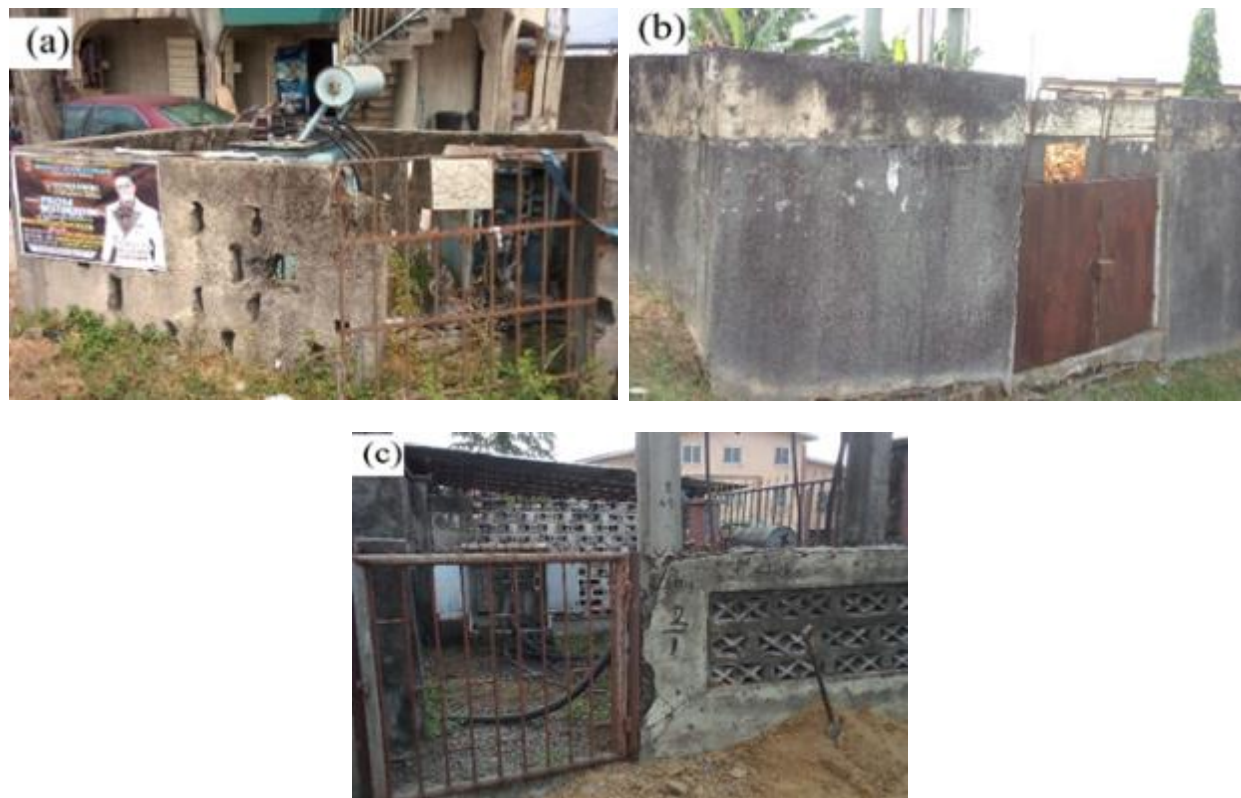
Figure 1 Locations Photos of Transformers (a) Ubeji (b) Ogunu and (c) Edjeba in Warri South Local Government Area, Warri Metropolis
