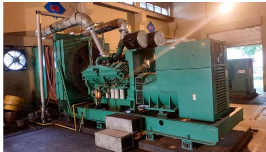
Figure 5 Generator Set 1000 kVA
